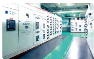
Smart Power Distribution Room
